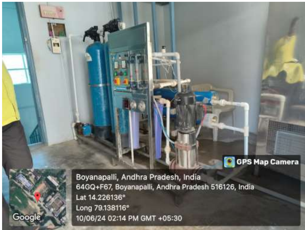
RO System water body management
