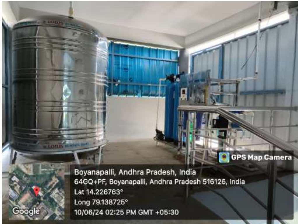
RO Water Storage Maintenance system
