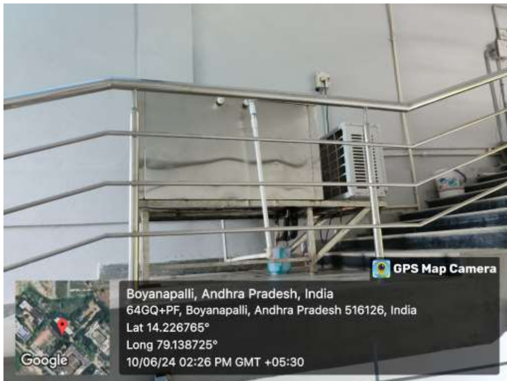
RO Water refrigeration maintenance System
